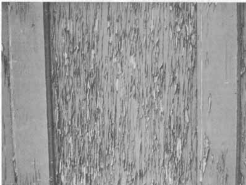
Figure 4—Early paint failure on plywood because of penetration of moisture into surface checks of plywood. M830013-6
