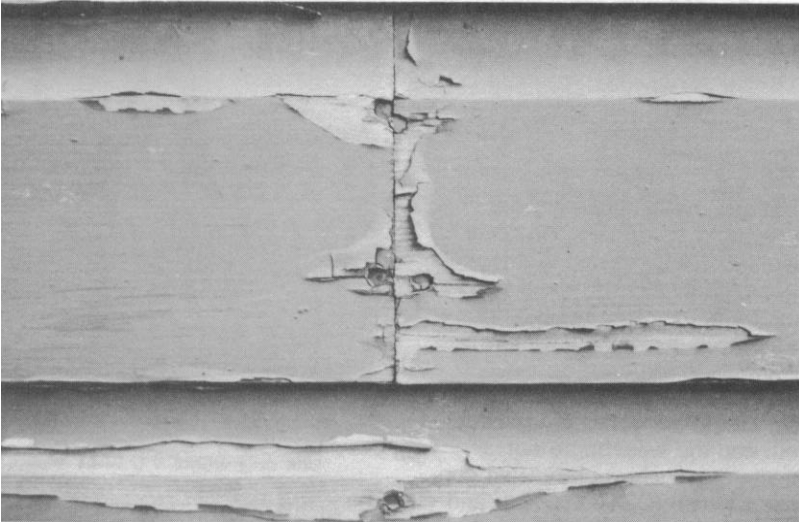
Figure 14 —Paint normally fails first around the ends and edges of a board. Liberal application of a water-repellent preservative can prolong paint life in these areas. M8330013-5
