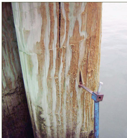
Piling in Charleston, South Carolina, damaged by salt exposure. This pile was located in a marina and subjected to frequent wetting and sea spray.
