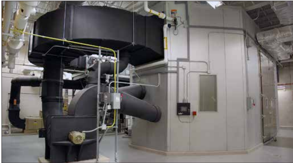
CARWASH test facility at the Forest Products Laboratory.
