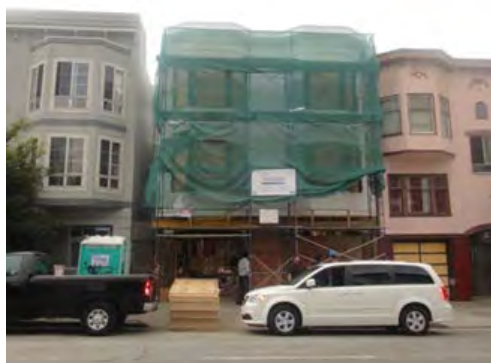
Figure 1. Soft-story woodframe building in San Francisco, California undergoing voluntary retrofit.
