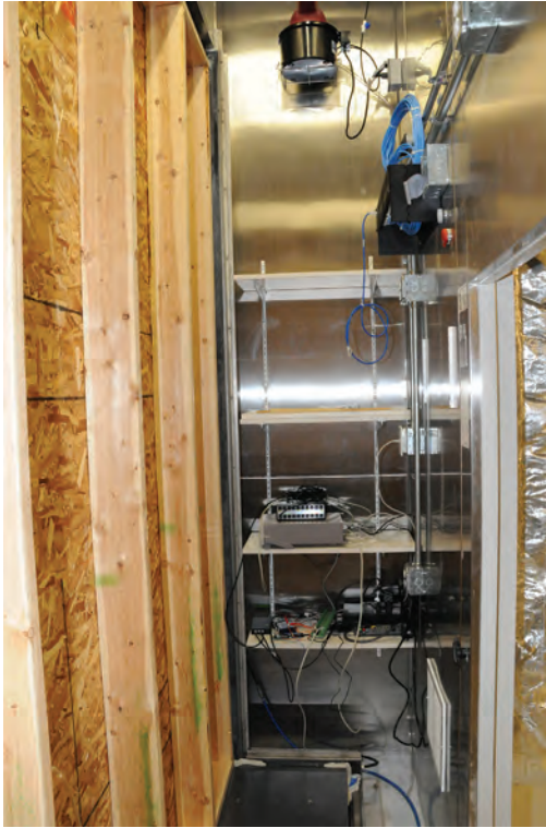
Figure 3 Small indoor chamber in CARWASH.
