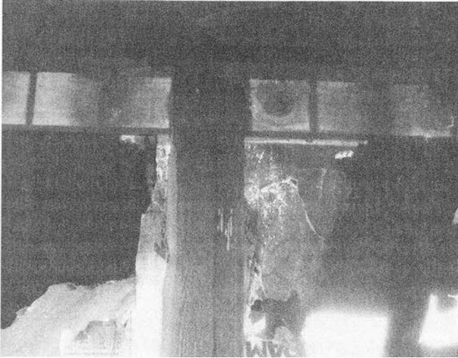
Figure 6.4 Fire-damaged timber floor beam
