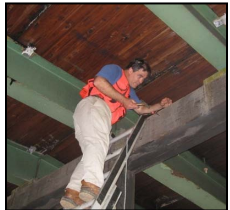
Figure 3 – Nondestructive assessment included resistance micro-drilling (top) and stress-wave timing (bottom) in the columns and cap beams.
