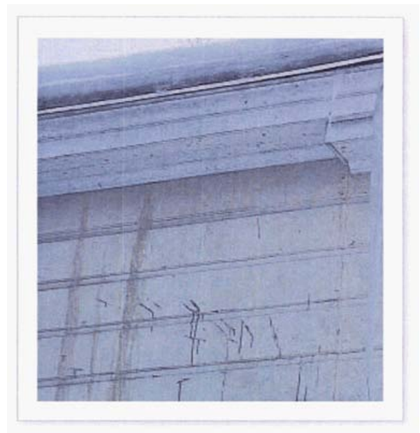
Figure 4 - Ice dam on roof and gutter. The resulting water intrusion into the wall and behind the siding often causes run-down extractive bleed.
