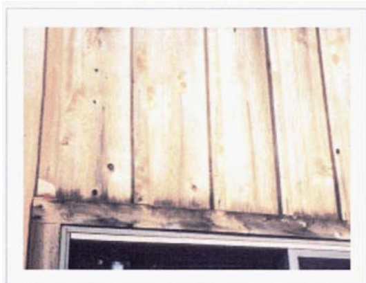
Figure 3 —Extractive bleed from end-grain adsorption of water. Note the fasteners have also caused iron staining.
