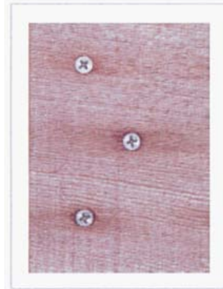
Figure 6—Extractive bleed around stainless steel fasteners.
