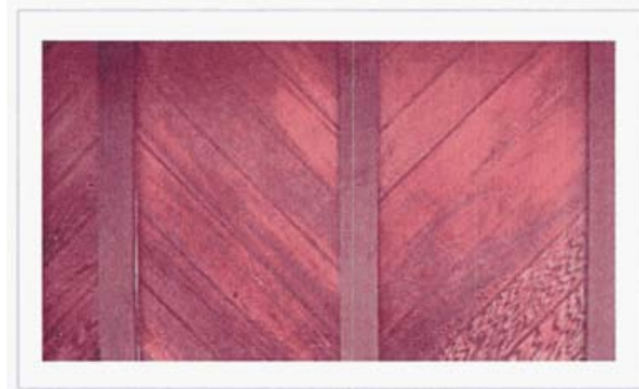
Figure 5 - Uneven extractive bleed on siding.
