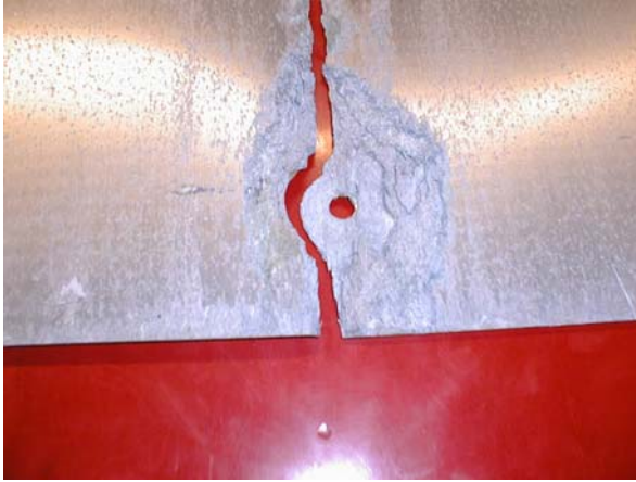
Figure 1: Failure of an aluminum traffic sign that was attached to ACQ-treated wood with a stainless steel fastener. Photo courtesy of WISDOT.
