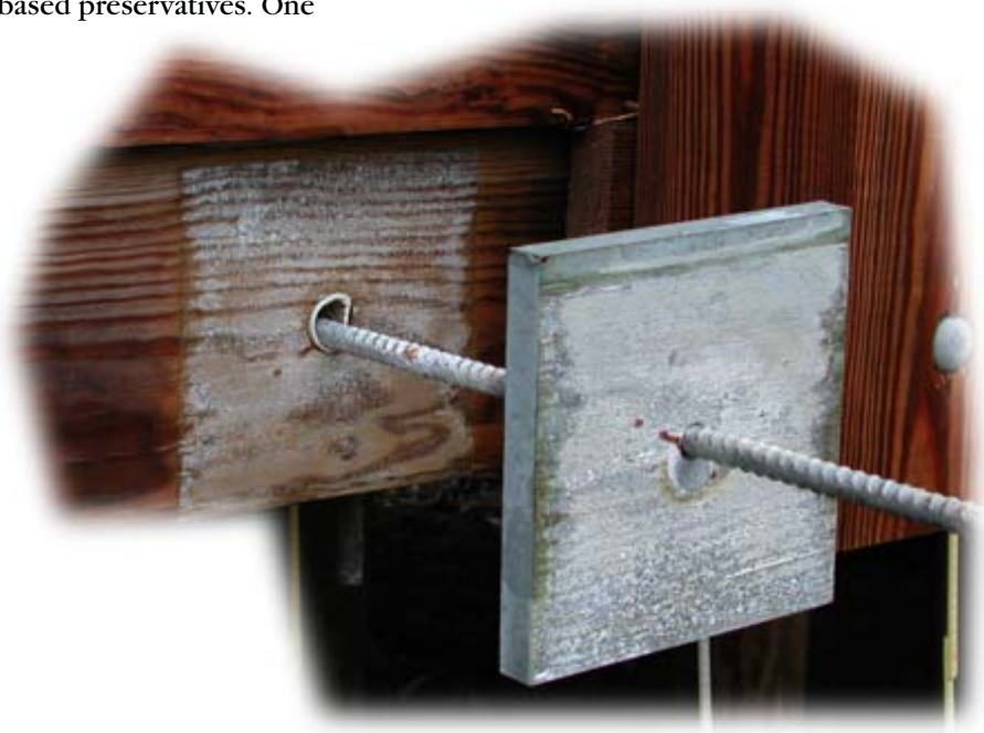
Figure 10—This metal plate used in a stress-laminated bridge constructed with preservative-treated wood shows the early signs of corrosion.— Photo courtesy of James Wacker
