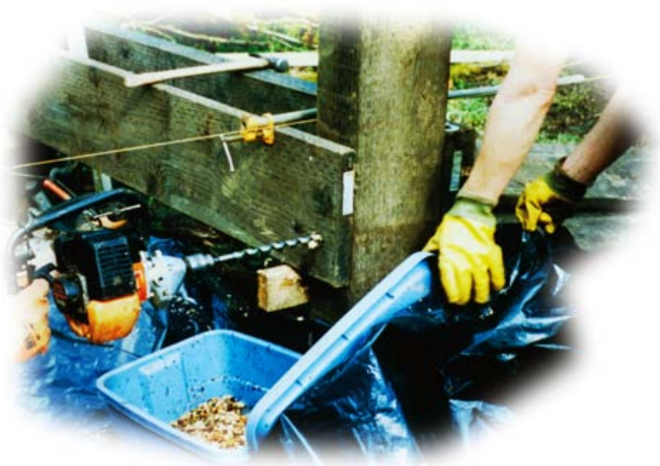
Figure 9—A tub can be used to collect sawdust when drilling preservative-treated wood. Collecting debris during construction helps to minimize environmental impacts.
