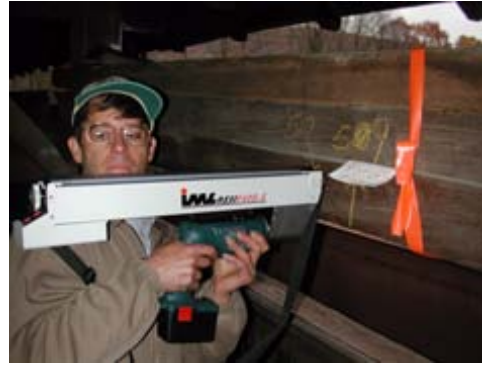
Figure 9. Using a resistance-drill to locate interior decay in an upper a chord member.
