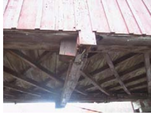
Figure 5 – View of floor joist system from below. (Note the retrofitted tie beam fastened with canted rods that imposed enough horizontal force to damage the lower post relish.)
