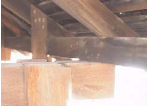
Figure 2 – Assembly of truss posts and upper chords, tie beams, and rafter / sills
