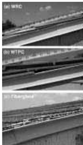
Figure 2. — Side view of shingles installed in 2001 at Valley View test site in Wisconsin. Ruler shown in inches.
