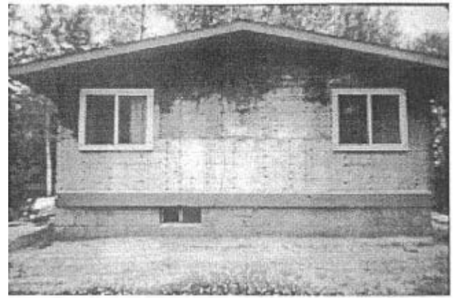
Figure 5. —Mold and decay caused by insufficient roof ventilation and lack of vapor barriers in the ceilings.
