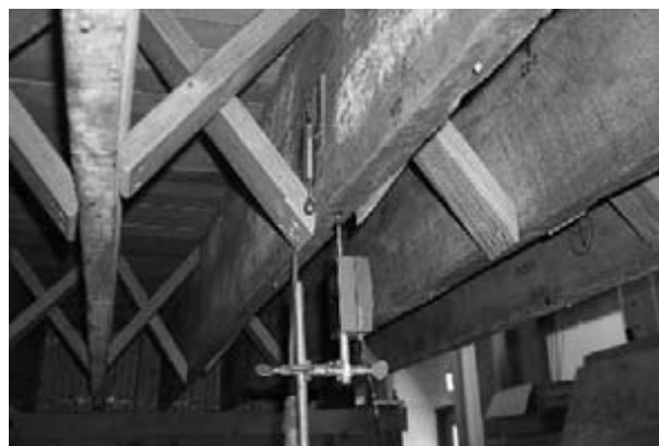
Figure 1. Typical wood floor system constructed with solid-sawn wood joists, cross bridging, and deck boards
