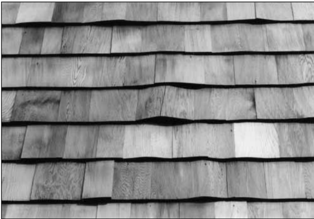
Figure 7. Buckling of shingles installed with insufficient gap.
