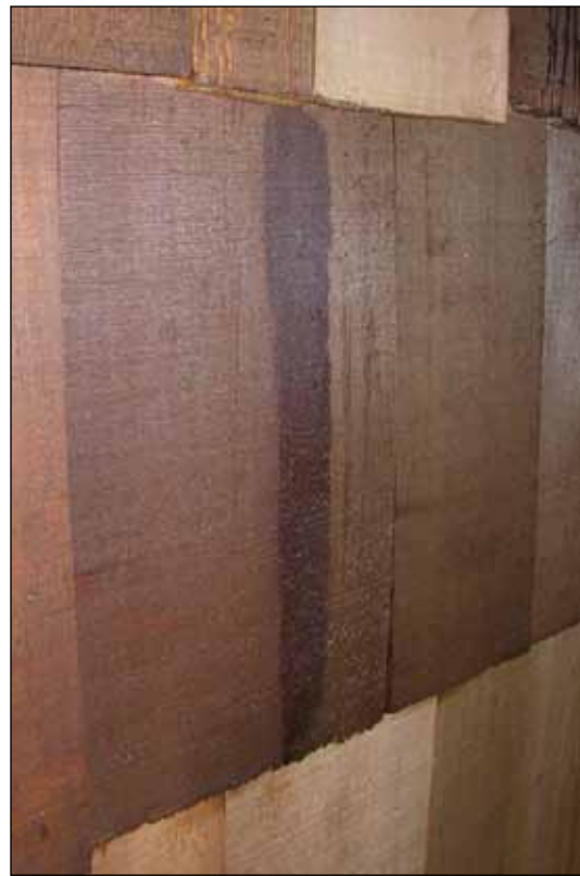
Figure 16. An example of a lap mark from improper application of a semitransparent stain.
