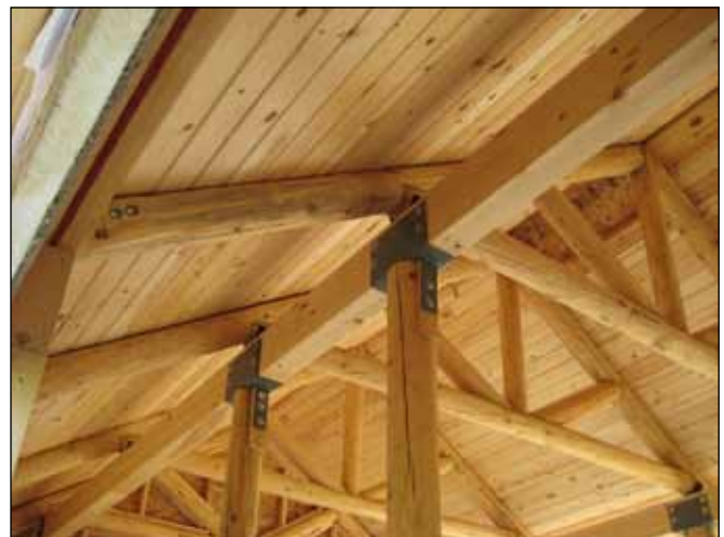
Figure 4. Interior view of the small-diameter log (SDL) structure, glulams, and tongue-and-groove decking.
