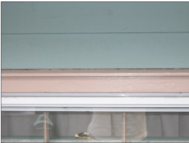
Figure 3—Wood drip cap, atop window head casing, installed in shingle-lap fashion with redcedar trim and without caulk. In this example, there is no metal head flashing over the wood drip cap and behind the siding. Water intrusion between the drip cap and the siding could be expected if this detail were exposed to significant wind-blown rain. A modest 0.3 m (12 in.) roof overhang on this single-story home evidently provided adequate shelter from wind-blown rain. This is the same window shown in Figure 1B.
