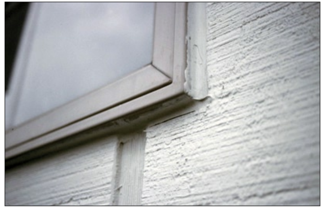
Figure 8—A perimeter sealant joint around a contemporary flanged window. The joint is of appropriate width at 6 mm (0.25 in.). The joint had been in service for roughly 3 years when photo was taken. Joint is mostly intact, but some adhesion failure is evident at lower right corner. As is common in residential construction, neither bond-breaker tape nor sealant backer was used. Joint failure is likely the result of three-sided adhesion, an unprimed siding edge, and other-than-ideal sealant width–depth ratio (sealant depth exceeding width).
