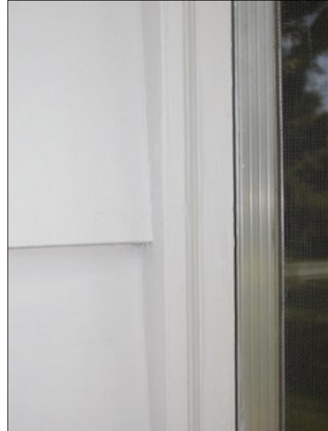
Figure 1A—Painted red cedar bevel lap siding butted tightly to window jamb casing without caulk. Photograph taken summer 2005 on ranch-style home constructed in 1960.
