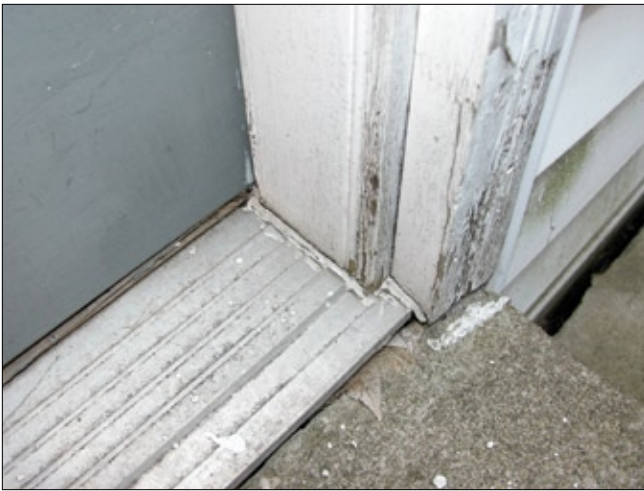
Figure 13A—A failed fillet caulk joint between the ribbed aluminum sill and the pine jamb and jamb casing of a contemporary exterior door. The ribs retard drainage off the aluminum sill. The short length of fillet that runs parallel to the ribs also retards sill drainage and does so at a critical location.
