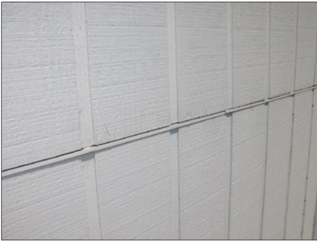
Figure 10—Metal Z-flashing at a horizontal joint in plywood panel siding. The second-story (upper) plywood panels should have been installed approximately 3 mm (1/8 in.) higher than in this installation. This would have provided more adequate drainage space between their lower edges and the horizontal leg of the Z-flashing (a paint bridge between the siding and the Z-flashing can be seen at the left-most groove in the photo). Well executed Z-flashing (without caulk) has proven effective at joints like the one shown here.
