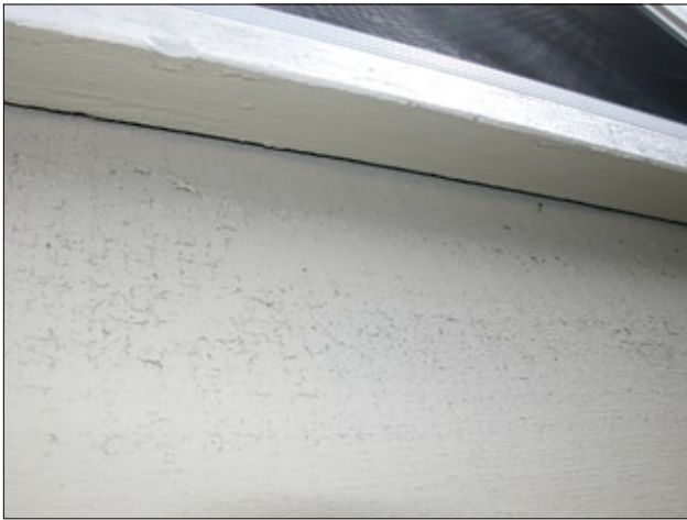
Figure 2—Wood siding shingle-lapped with an outwardly sloped wood window sill without caulk. Photograph taken in summer 2005 on a 1½-story home constructed in 1916.
