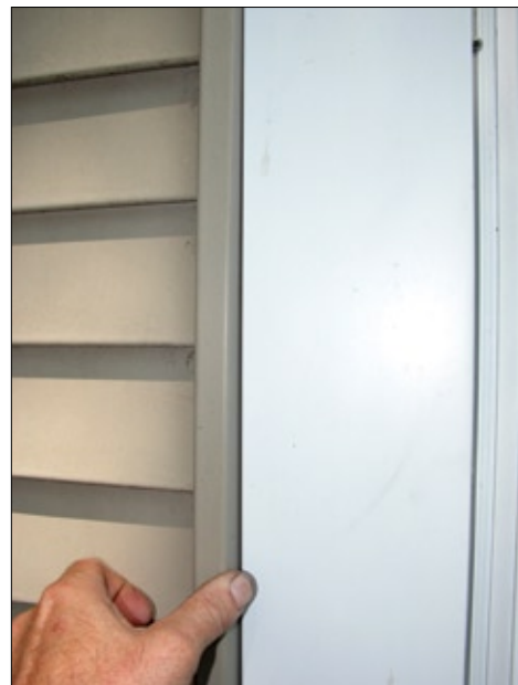
Figure 4B—Interface of vinyl siding J-channel receptor and aluminum window jamb trim. Outward thumb pressure against the J-channel reveals that there is no caulking between the J-channel and the jamb trim. This is consistent with installation guidance available from the trade association for vinyl siding. This installation was about a decade old when the photo was taken and had performed acceptably.
