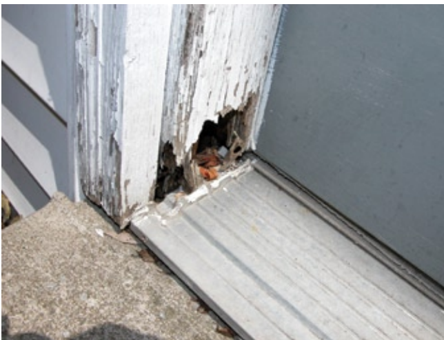
Figure 13B—Extensive jamb decay in a contemporary exterior entry door. The decay was in all likelihood exacerbated by the short length of fillet joint that blocked drainage at the outside lower edge of the jamb.
