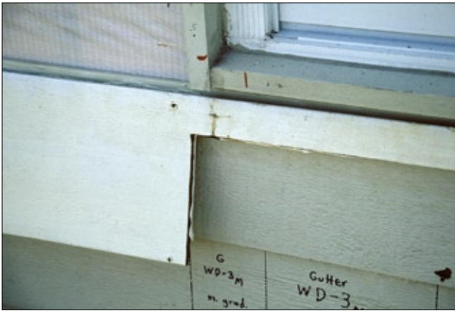
Figure 9—Water staining on the back surface of hardboard siding on a test building. Leakage, although modest, occurred in 29 months of service and was determined to be through sealant joints. The sealant used in this installation met the requirements of ASTM C 920. None of the joints showed outward indication of failure. Subsequent laboratory testing indicated that the window unit, although not of the highest quality, was not the leak source. Sealant joints were a combination of bedded, butt, and fillet. At fillet joints, sealant adhesion at joint root was a likely contributor to failure. The building was in Florida where conditions at joint installation were hot and humid. These conditions would accelerate cure of the polyurethane sealant used. “Skinning” of the sealant before tooling was therefore also a plausible contributor to joint failure.
