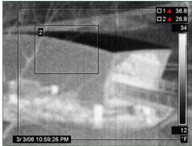
Covered bridge infrared monitoring can prove to be very beneficial in night time applications.
