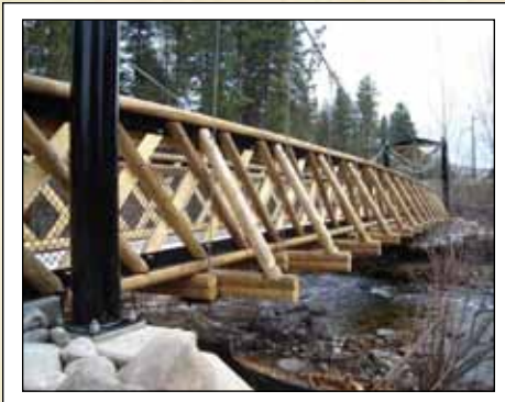
The Rattlesnake Creek bridge near Missoula, Montana, was built using 6-inch-diameter lodgepole pine from a forest in Idaho to demonstrate the effective use of trees killed by the pine bark beetle.
