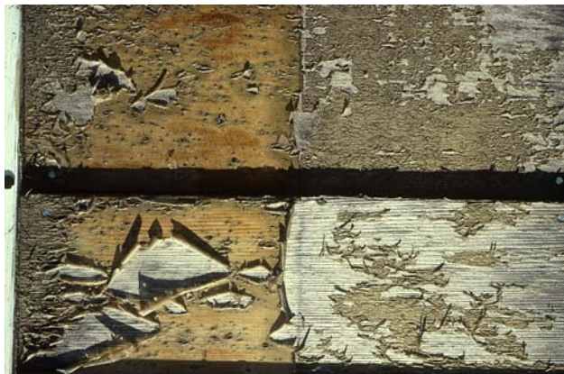
Figure 1 – Coating failure on wood.
