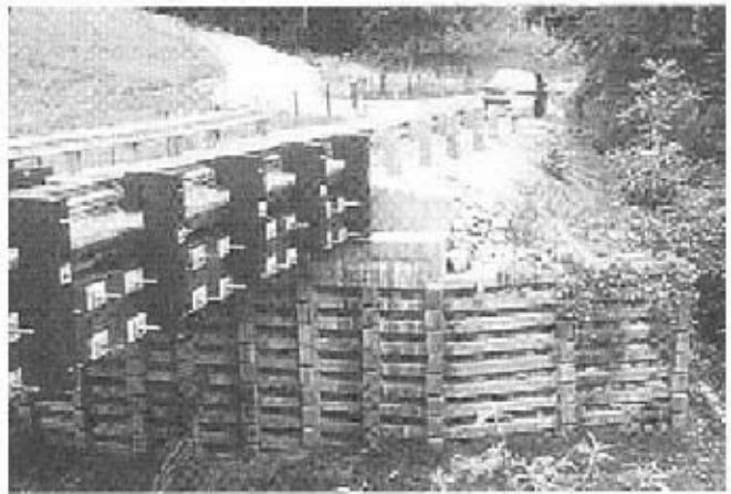
Figure 4.1. – Timber bridge in Jackson County West Virginia containing 1650f-1.4E machine stress rated oak decking.
