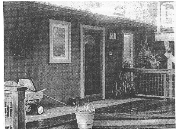
Figure 8. ~ Wide overhangs on this structure protect the cladding and penetrations (windows and door) from rainfall. Note the dry deck boards near the house, and the wet deck boards away from the house.
