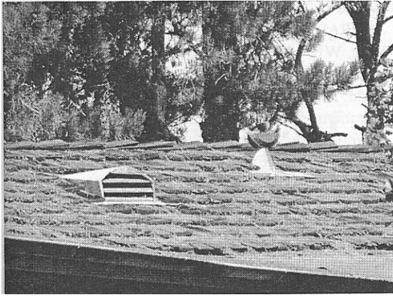
Figure 7. ~ An example of a dormer-type through roof vent that would be vulnerable to both wind-driven rain and flames and embers from a wildfire. Debris from nearby pine trees and the untreated shake roof also pose significant problems for this structure.
