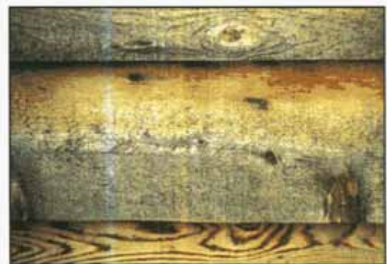
Figure 5—Mildew on wood siding.
