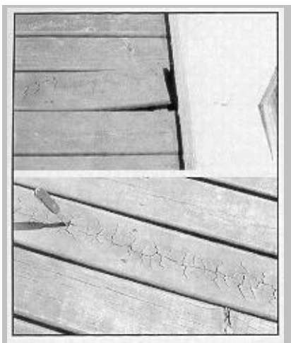
Figure 8—Warping (top) and excessive surface degradation (bottom) resulting from juvenile wood.
