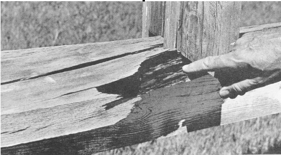
Figure 2. Closeup view of decayed untreated window unit frame. Window unit fell apart after 6 years' exposure.
