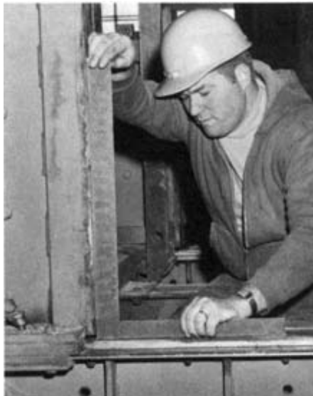
Figure 53.–Check the knee and head-block base for a 90-degree angle with a carpenter's square.
